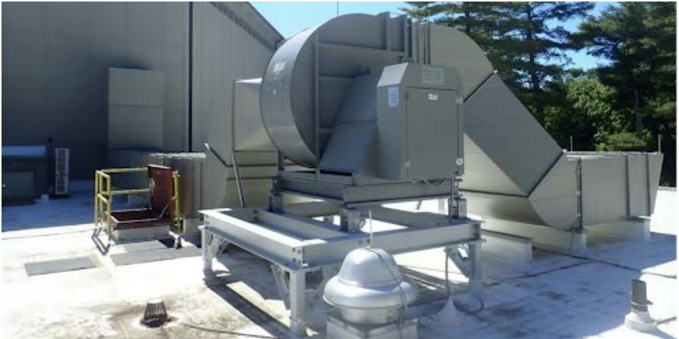
New quiet ventilation fan on roof of amenities building behind the Koussevitsky Music Shed
