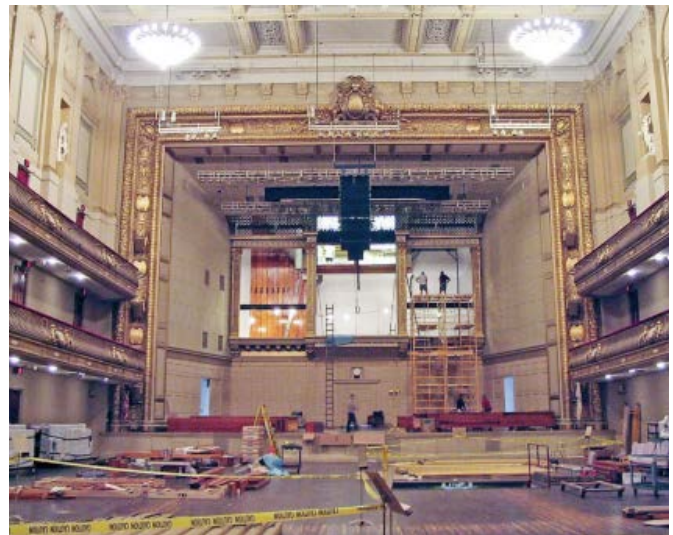
Pipe organ chamber exposed and bare, organ pipes on floor in foreground
