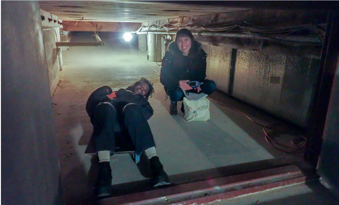
Acentech intern Jehan Diaz and acoustician Allie Lam in Ozawa Hall's underfloor air circulation spaces.
